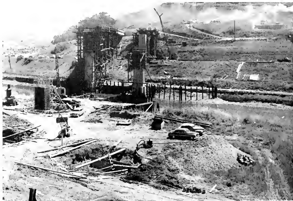
ABOVE—Looking southerly at Petaluma Creek Bridge and Overhead during construction. Channel must be kept clear for navigation at all times. On far bank is Northwestern Pacific spur line into Petaluma.
